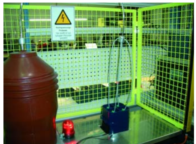
Figure 5: Every GIS18 is subject to intensive high-voltage testing prior to delivery
